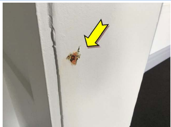
Photo 12. Interior, throughout, walls – lead-containing light green lower paint system.
