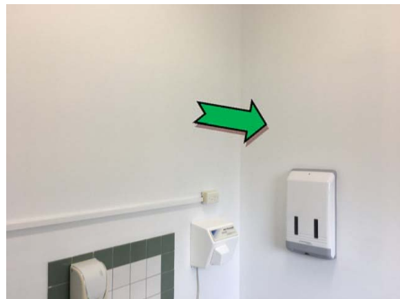
Photo 6. Interior, throughout, disabled toilet, wall lining – non asbestos containing fibre cement sheeting.
