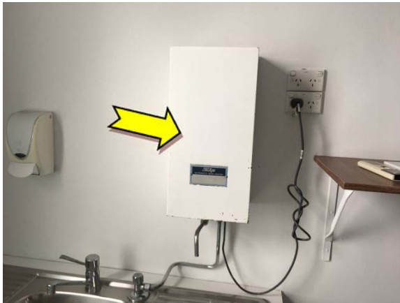
Photo 9. Interior, staff room, hot water boiler – suspected SMF internal insulation material.
