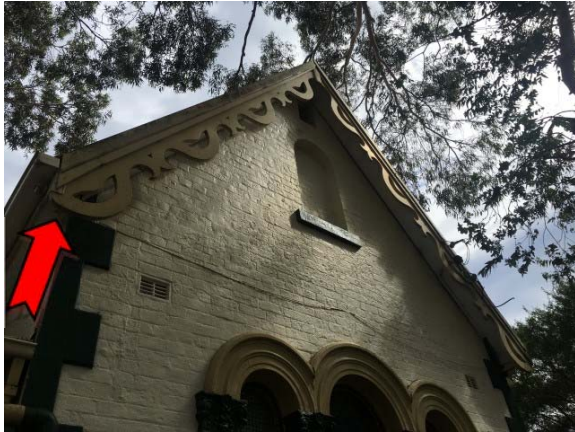
Photo 1. Exterior, throughout, eaves – suspected asbestos-containing fibre cement sheeting.
