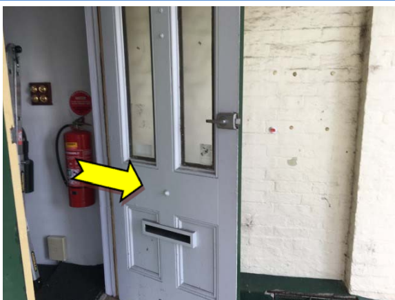
Photo 11. Interior, entrance lobby, door – suspected lead-containing grey upper paint system.
